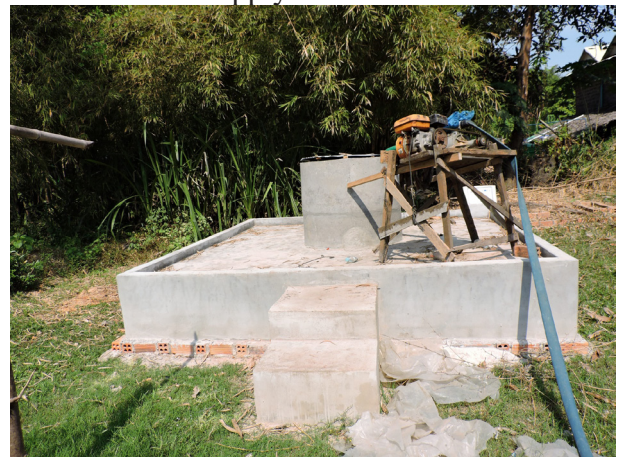
Figure 7: Deep drilled well for year-round water supply
